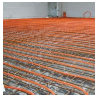
Industrial floor heating
