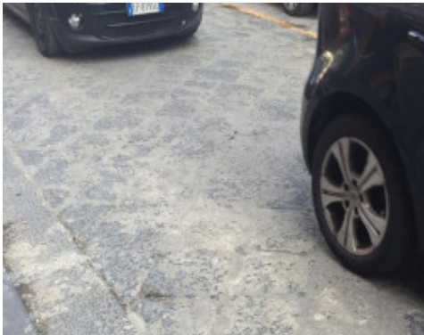
Stone paving spoiled with grouting remains
